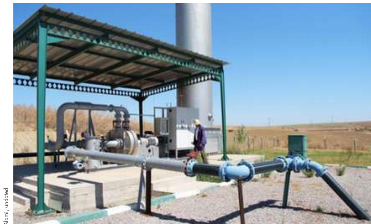
Figure 4.5: LFG collection system, Fès landfill, Morocco
