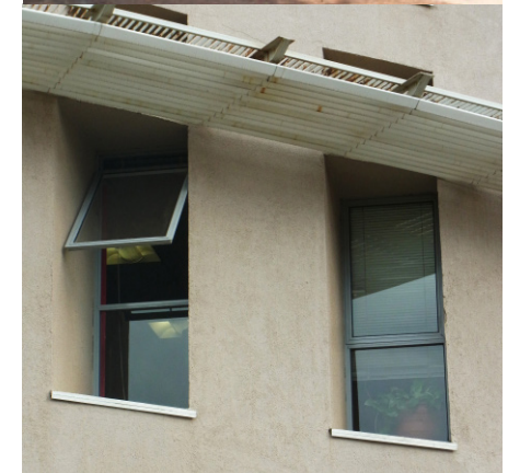
Appropriate Window to Wall Ratio and horizontal shading devices. © UN-Habitat / UMU (top); © UN-Habitat / Zeltia Gonzalez Blanco (bottom)
