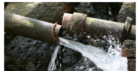
An average of 30% of water used in cities is wasted due to leakages in the distribution system © Pulpolux
