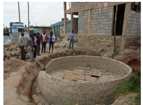
Biogas tank under construction in informal settlement where there is no access to sewer © UN-Habitat / Zeltia Gonzalez Blanco
