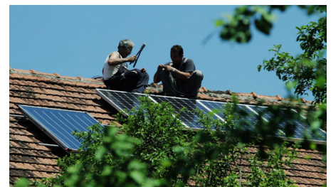
Installation of photovoltaic panels in the roof. Note: the limited losses allowed by orientation tilt and shading shall be the same than for solar water heating panels © UNDP
