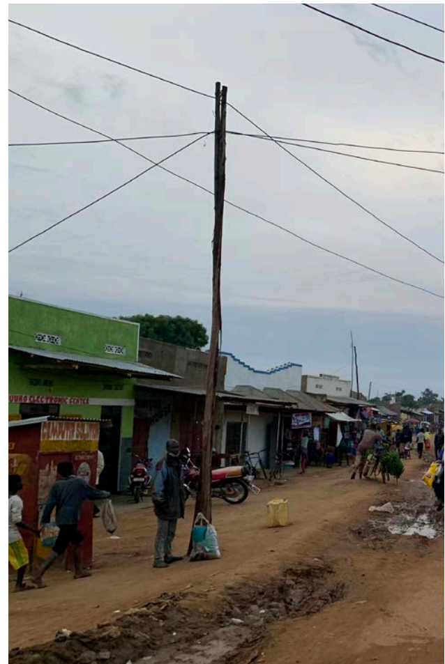
Fig.51: Informal Electricity Network in Base Camp
