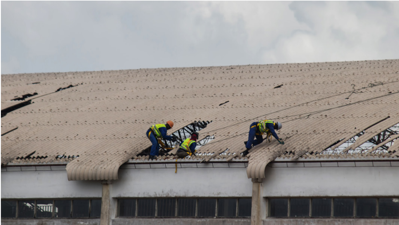
People fixing a damaged roof after a cyclone, Beira city, Mozambique © Shutterstock/MiroS Lav
