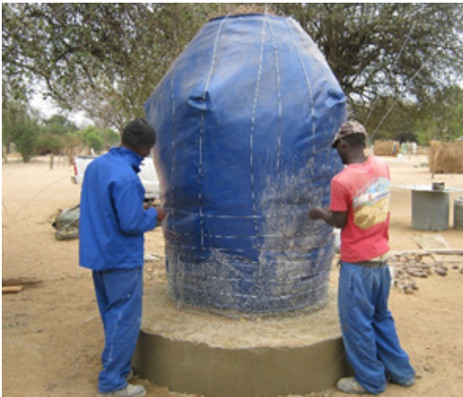
Figure 12: Improving water access through harvesting tanks in Chicualacuala, Mozambique. UN-Habitat, INGC
