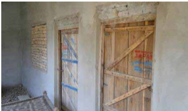
Figure 13: Poor quality door
