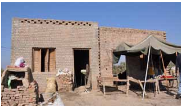
Figure 5: Katcha house, back wall collapsed
