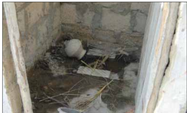
Figure 33: Latrine not maintained
