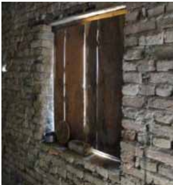
Figure 12: Poor quality window
