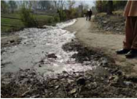
Figure 45: Village link road flooded due to lack of drain
