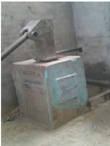
Figure 40: Afridev hand pump used in KP A good quality hand pump (KOICA project area)
