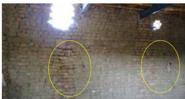
Figure 9: Improper location of girder
