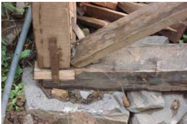
Figure 32: Non-compliant Dhajji house in AJK
