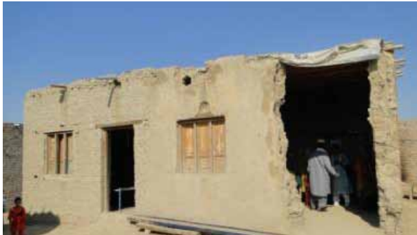
Figure 11: Misplaced girder led to collapse of wall
