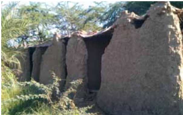
Figure 3: Adobe house destroyed by heavy rain
