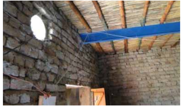
Figure 14: Walls not plastered, misplaced girder
