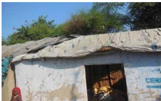
Figure 24: Sagging roof problem
