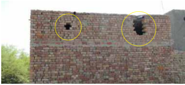
Figure 10: Need for PCC pads under roof drainage pipes
