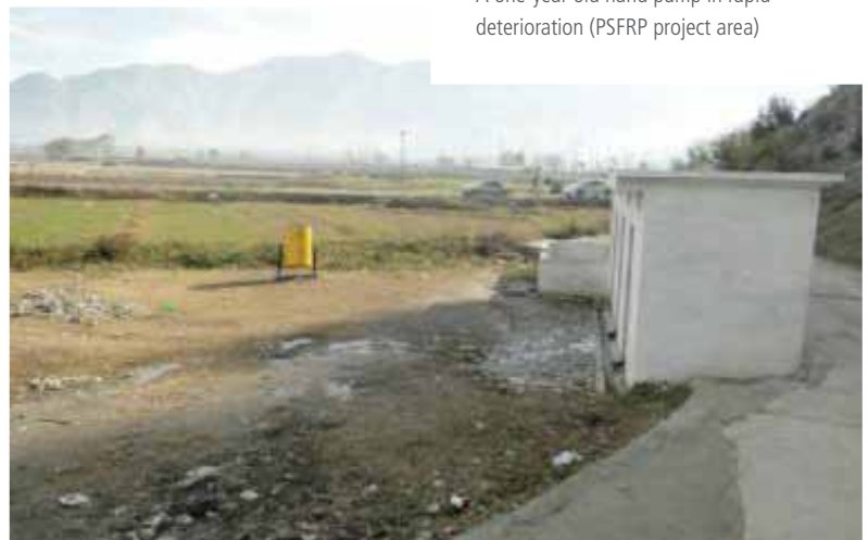
Figure 41: Washing pad and community bathroom was muddy and slippery. A PCC pad should have been placed in front.
