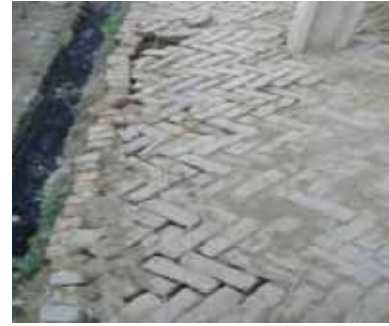
Figure 47: Village drain and pavement not maintained in a PSFRP project area
