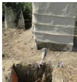
Figure 34: Unfinished septic tank and latrine
