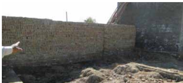
Figure 7: Collapsed house of fired bricks with mud mortar
