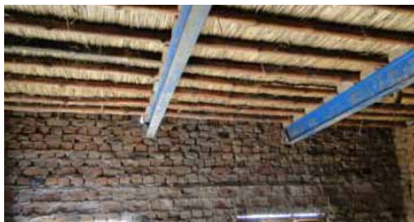
Figure 8: Poor workmanship, no PCC pads to support the girder
