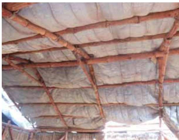
Figure 25: Roof frames too far apart
