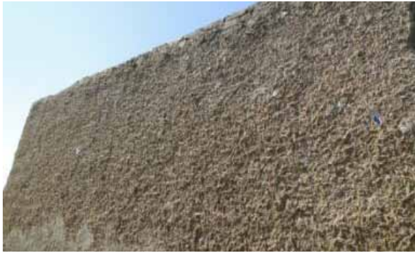
Figure 2: Adobe house, eroded walls
