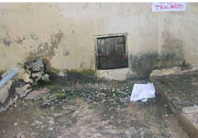
Figure 42. The small door through which the bucket latrine is emptied by a conservancy worker Photo © M. Oteng-Ababio
