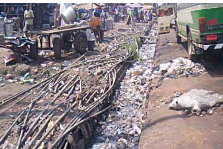
Figure 40. Such 'cat's cradles' of pipes make potable water vulnerable to contamination and increase water and revenue generation losses. Photo © M. Oteng-Ababio
