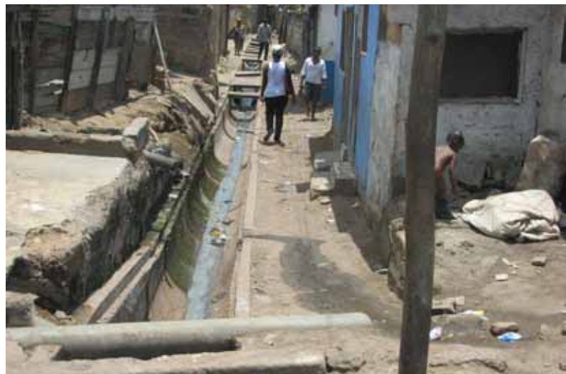
Figure 46. A drain fitted in the Nima upgrading programme Photo © M. Oteng-Ababio
