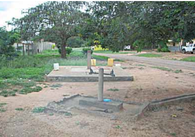
Figure 37. Public standpipe on the outskirts of Accra.
