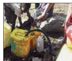
One of the public taps whose pipes have been removed and a garden hose attached.
