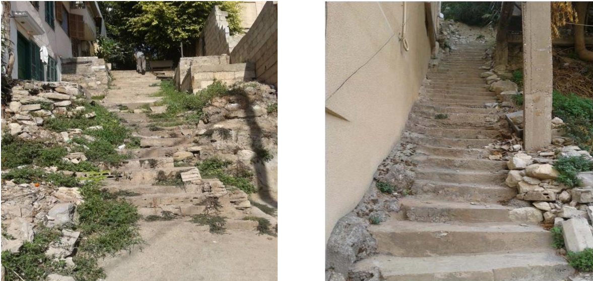
Photo 4: Conditions of the stairs in Karam El Zeitoun
