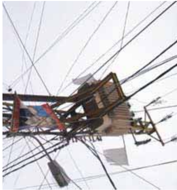
Electricity is provided in Sekke through a transformer installed by the Camp PC using financial contributions collected from dwellers
