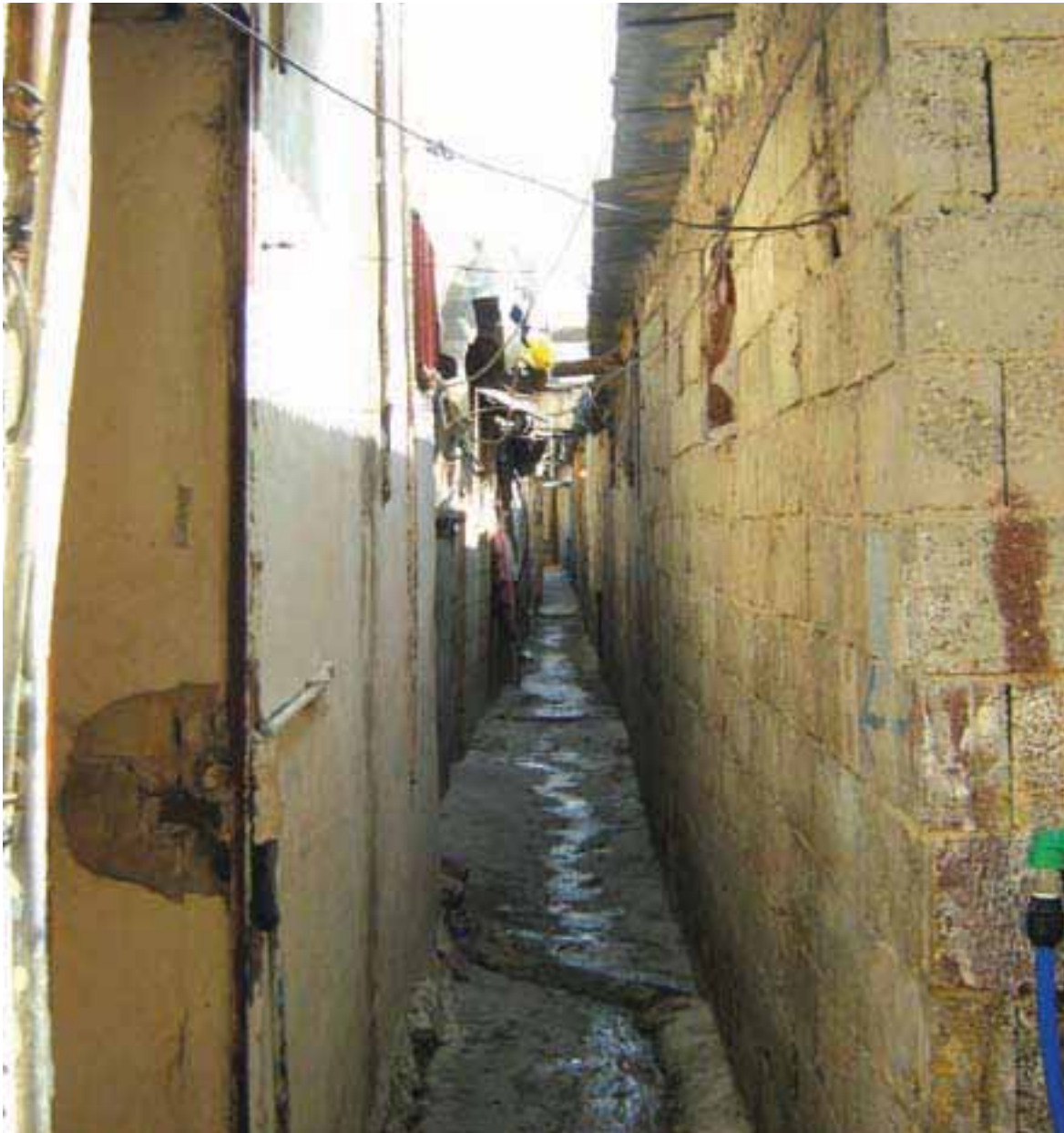
The width of alleys in Mouhajarin compromises lighting and ventilation conditions
