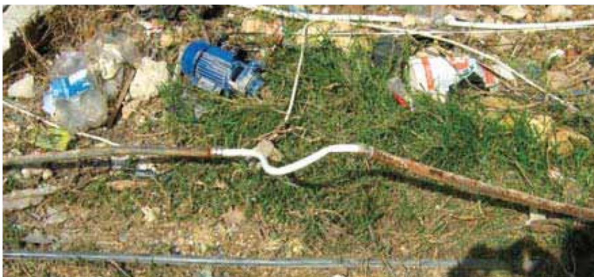
Basic methods of repairing water networks by replacing only the damaged parts, Jabal el Halib AA around Ain el Helwe Camp
