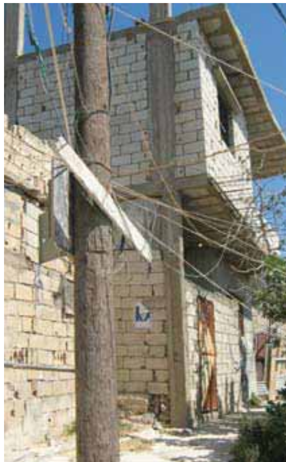
Basic methods for retaining loose and unshielded electricity cables in Hay el Wadi, Mieh Mieh AA
