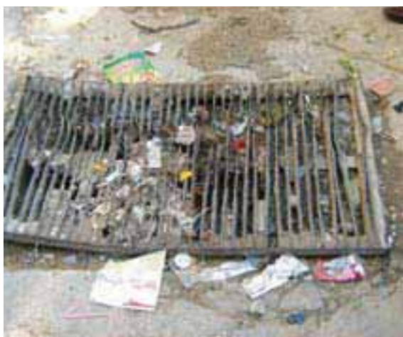
Blocked and damaged water drains in Bustan about Jamil
