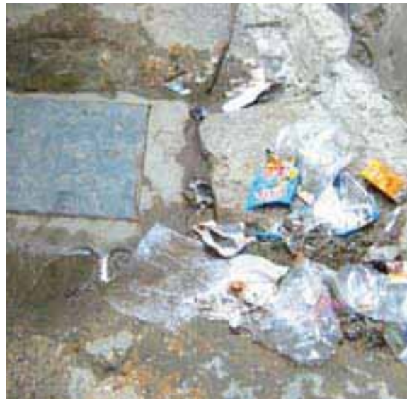
Most roads in Tawari are in need of rehabilitation and asphaltting
