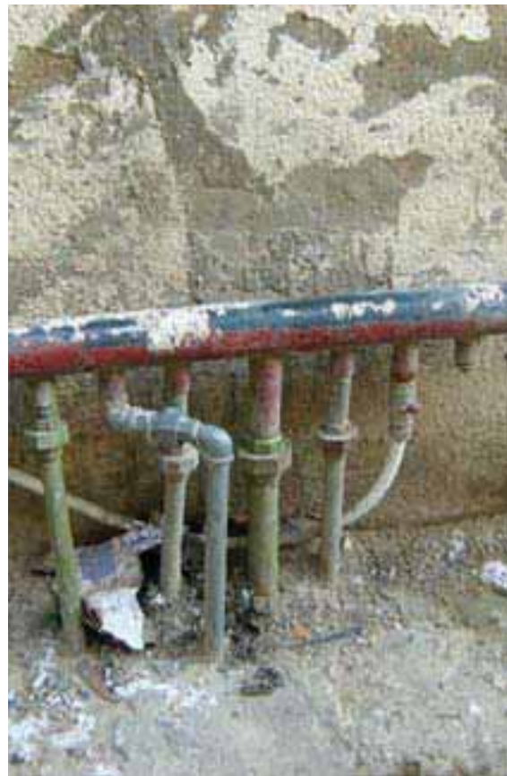
Collective water manifold installed by dwellers in Bustan about Jamil
