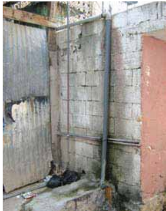
Steel pipes connected by dwellers for water provision in Baraksat
