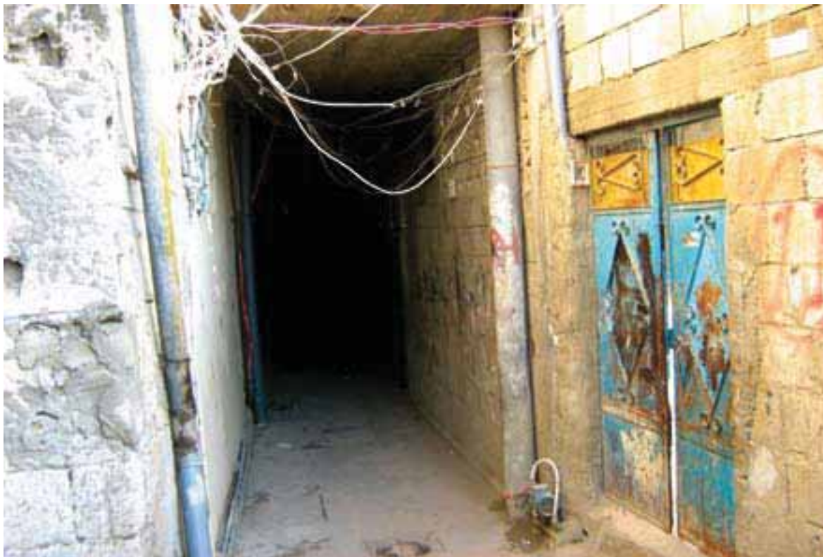
Informal electricity hooking in Bustan about Jamil
