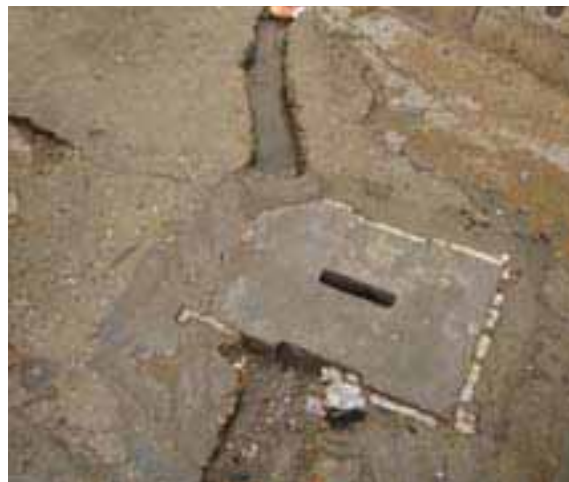
Basic drainage methods implemented by dwellers in Sekke to mitigate rain water flooding
