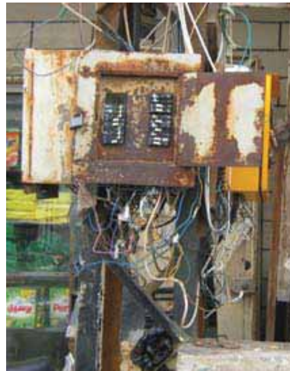
Ad-hoc connections to electric distribution boards, which replaced EDL meters, in Tawari
