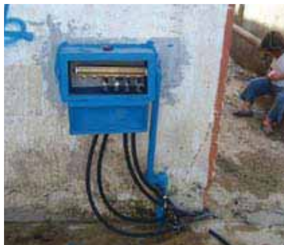
Collective water manifolds installed by UNRWA and UNICEF after the conflict in NBC AA (Source NBRC)
