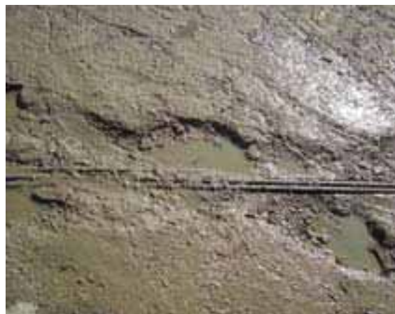
Partially exposed water network in Bustan el Kods
