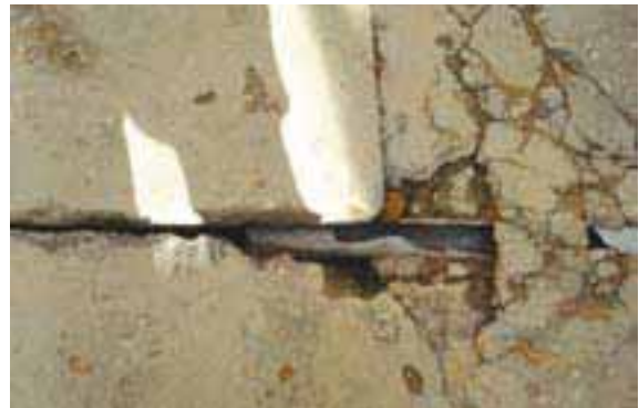
Damaged sewage pipes in Bustan el Kods
