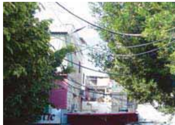
Water provision in Hay el Sohoun is compromised by the ad-hoc electricity connections (Note partially repaired cables)
