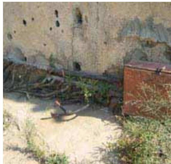
One collective manifold installed by UNICEF at the entrance of Tallet el Mankoubin provides water to all houses in the AA
