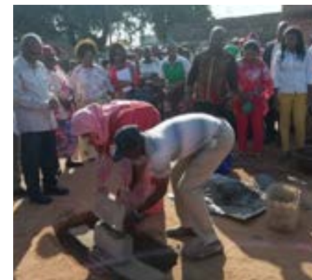
UN-Habitat Executive Director and the Mayor of Maputo launched the first stone of the construction that aims to improve a public space in the Bairro de Maxaquene D. © UN-Habitat Mozambique
