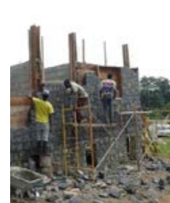
Construction of the houses- Resettlement of the Roça Sundry Community –'Terra Prometida' - The Island of Principe © UN-Habitat Principe
