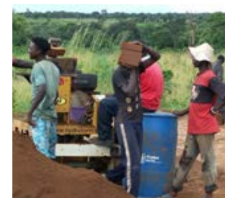
Making Soil stabilized bricks for low cost house in Mayukwayukwa © UN-Habitat Zambia
