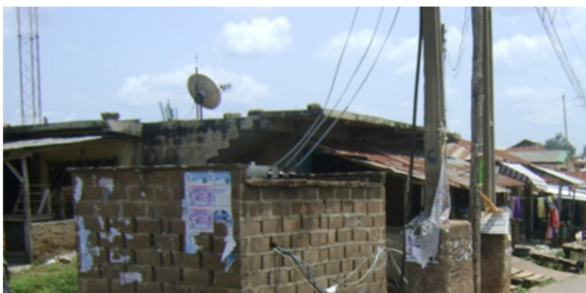
Plate 15: An 11KVA transformers in the Ede Planning Area
