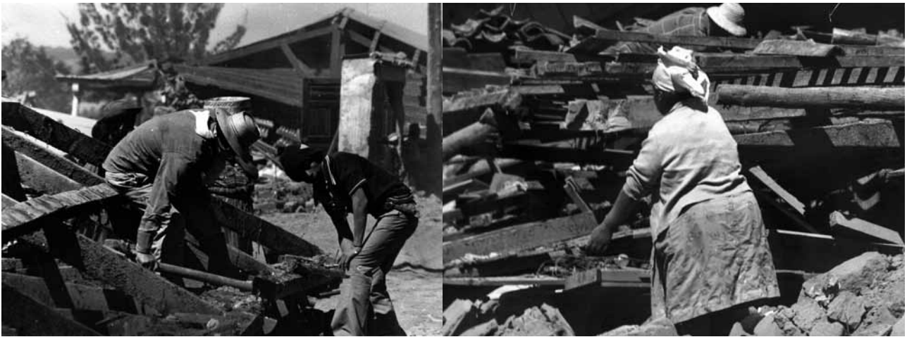
Families salvaging materials and beginning reconstruction 5 days after the earthquake Photos: Ian Davis
