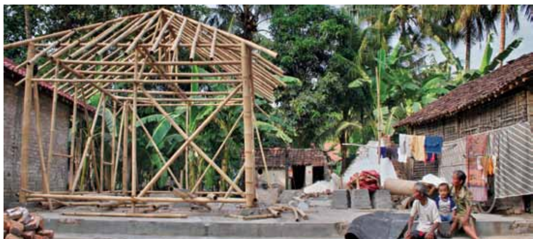
A transitional shelter built on the site of a destroyed house Photo: IFRC
