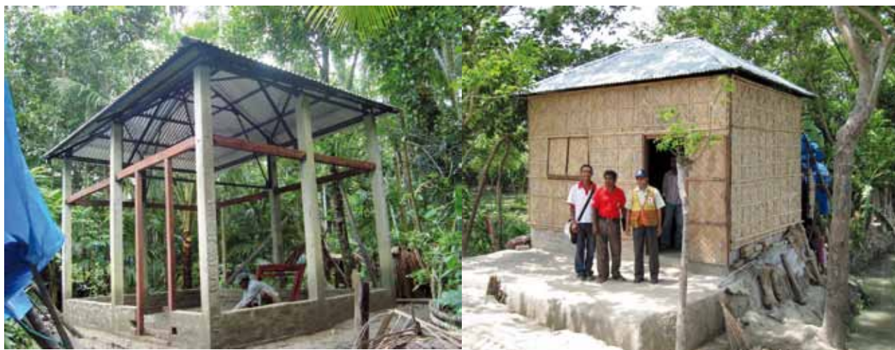
The core shelters were built by contractors and selection of families was through a lengthy transparent process Left shows the frame of the structure Photos: Xavier Génot, IFRC
