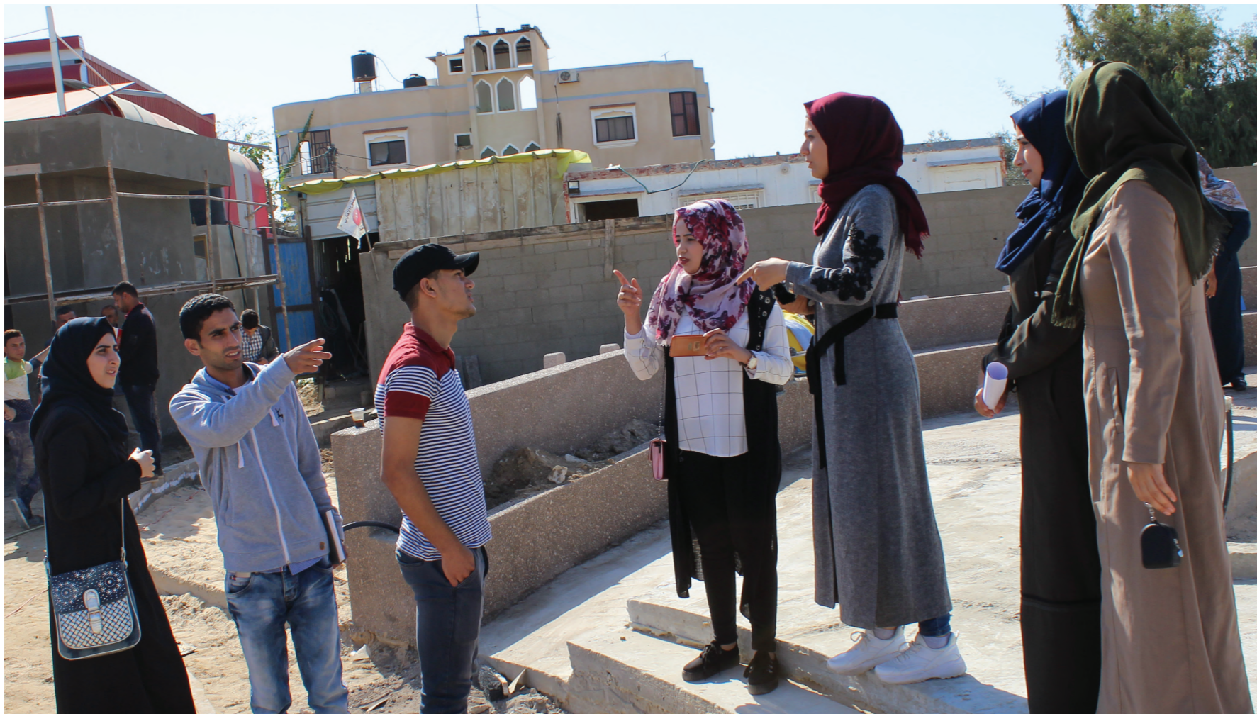
Men and women during construction of public space in Khan Younis © UN-Habitat
