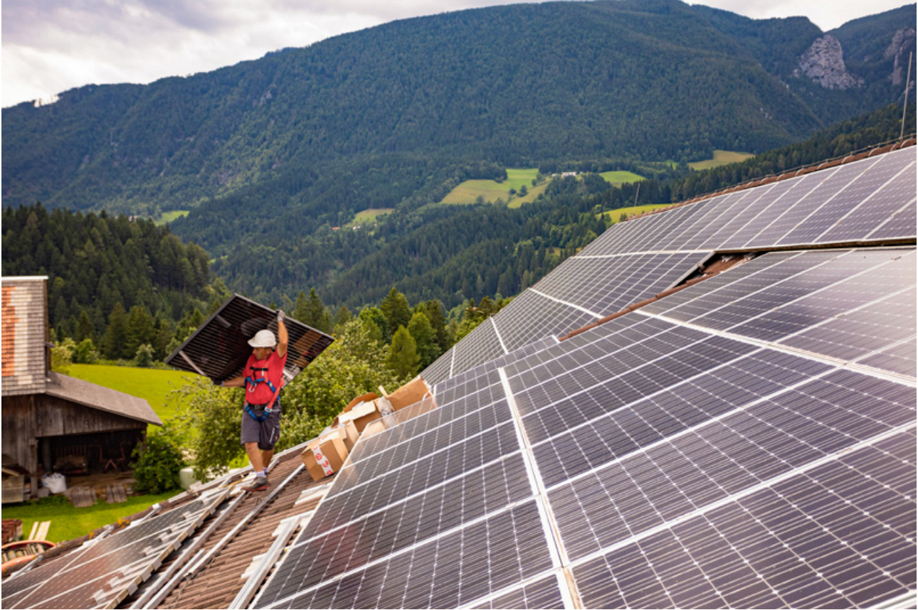
Photo 10 Installation of solar panels at the Luče energy community, Republic of Slovenia
