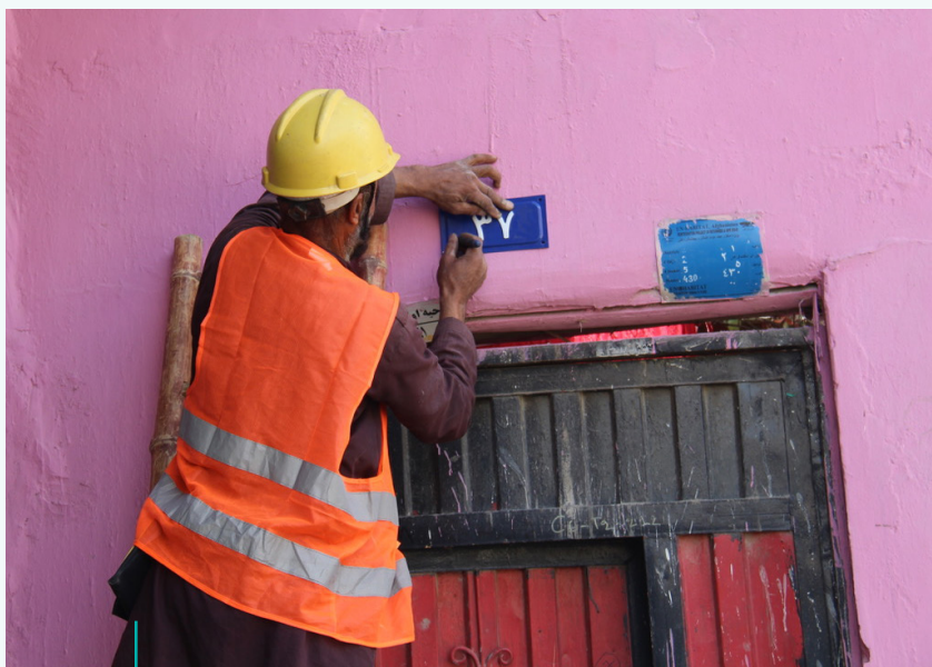
As part of the programme to regularize urban informal settlements, a worker installs a house number above a door in Kabul ©UN-Habitat/ Afghanistan
