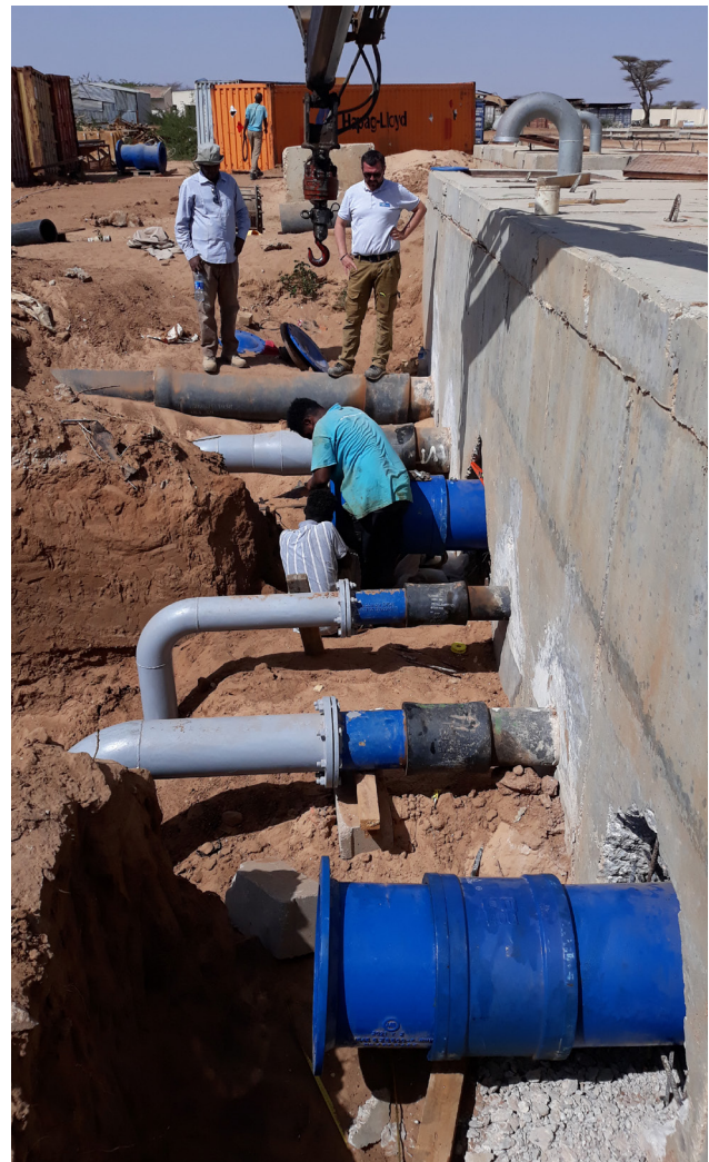
Connection of different wellfield collector pipes to the connection chamber at the new pumping station
