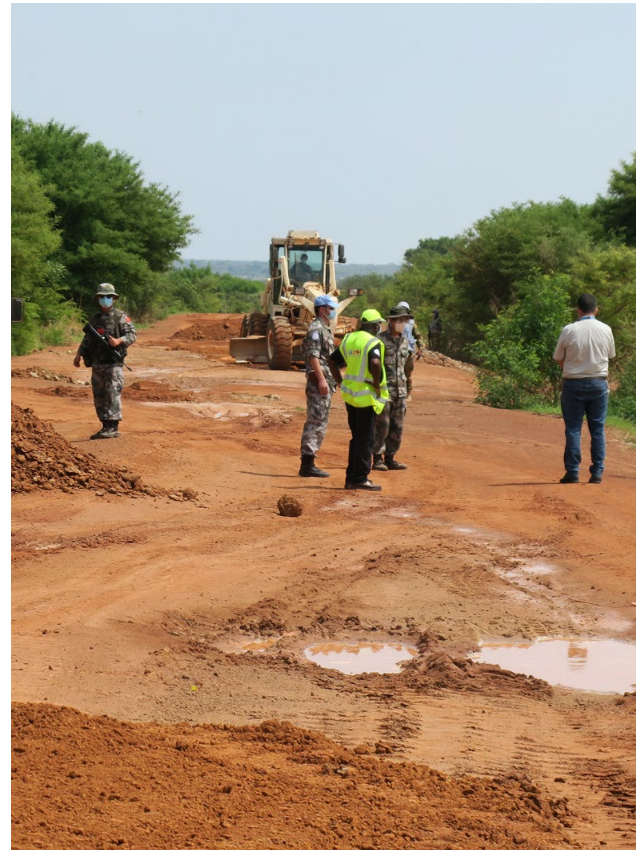
Figure 25: Repairing damaged roads for unhindered access to remote areas in South Sudan is a priority for UNMISS ©United Nations Mission in South Sudan (UNMISS), 2020
