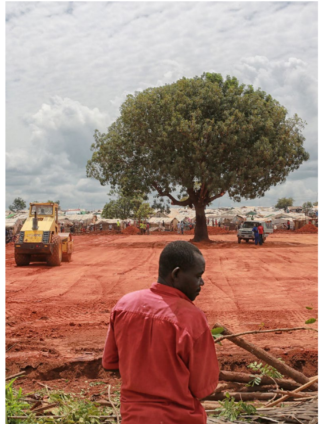
Figure 49: Spatial upgrading of a United Nations IDP Camp in South Sudan by UNMISS ©United Nations (UNMISS), 2017
