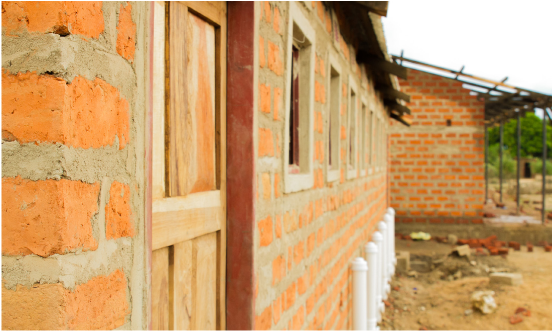
Red pan brick building for a classroom and toilet construction. © Shutterstock/ FANKS
