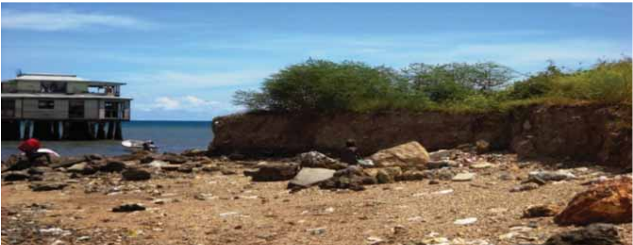
Eroded section of Koki seawall Photo © Auka, J., 2013
