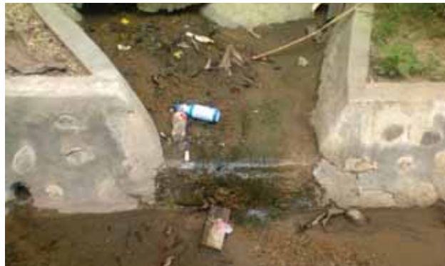
Drains blocked with soil and other waste materials in the Gordens Area Photo © Goiye, B., Kioma, T., Bobora, N., Bomai, A. and Kamaso, D. (2012)
