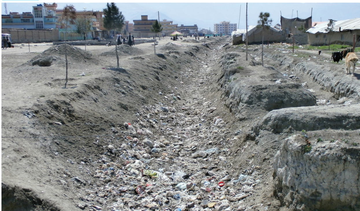
FIGURE 43 ROADSIDE DITCH FILLED WITH SOLID WASTE
