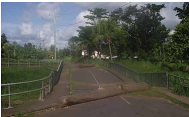
Lifeline bridge damaged at Leone. Photo © UN-Habitat / Bernhard Barth
