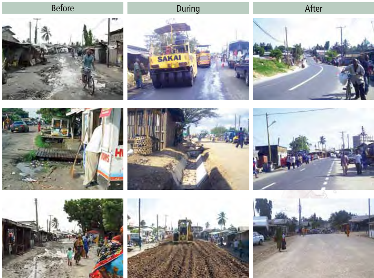
Before, during and after Phase I of the Community Infrastructure Upgrading Programme Photos © CIUP
