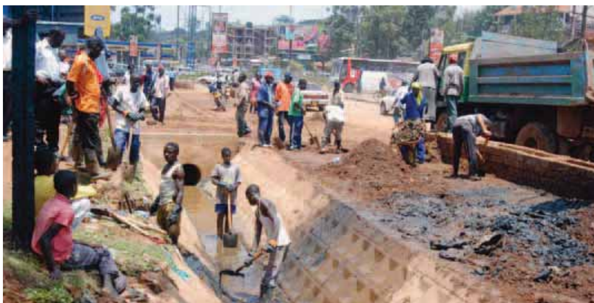
Kampala City Authority workers clear drainage along the Mulago-Kalerwe Road
