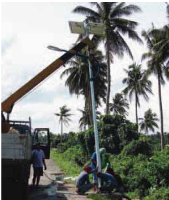
Installation of a solar-powered street light along Diversion Road in Sorsogon, Philippines © UN-Habitat/Joselito Derit
