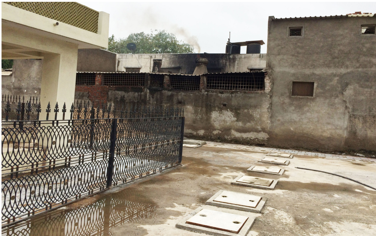
Decentralized waste water treatment system in Rajkot, India. © Earl Kessler
