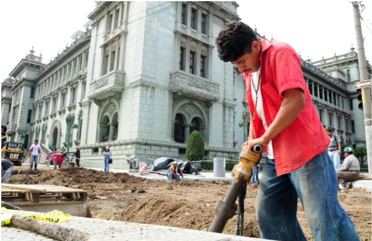
Public works in Sixth Avenue, zona 1, beside the National Palace, Guatemala City, Guatemala. © Maria Fleischmann/World Bank
