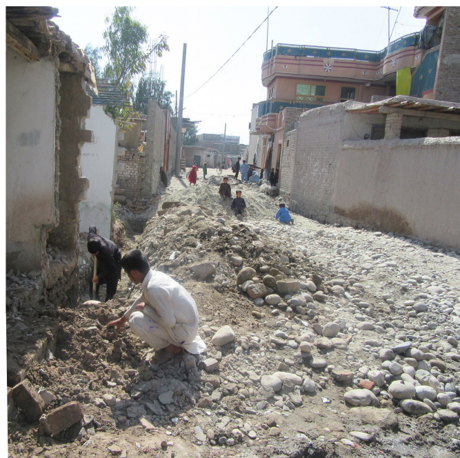
Picture 26: Unpaved streets, Qasamabad Damankalil
