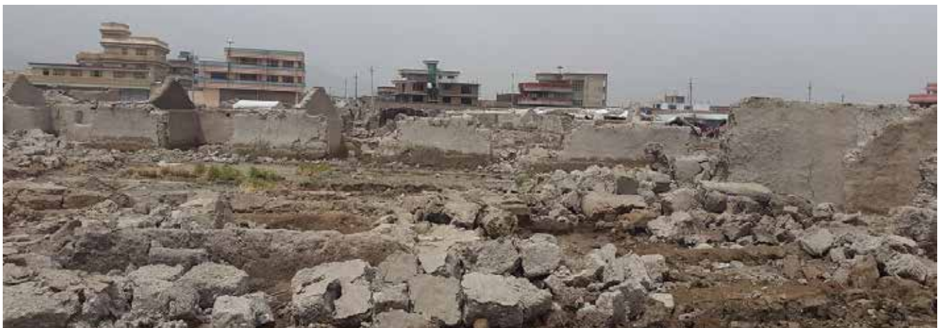
Picture 12: Informal housing in disrepair, Charmane Khossain Khail
