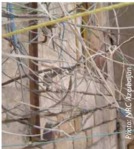
Wiring before upgrade
