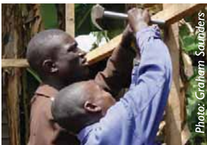
Families were trained to construct their shelters, but around 70% hired others to build.
