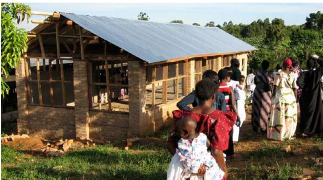
Ground breaking day celebration of a new poultry house in Masaka © UN-HABITAT
