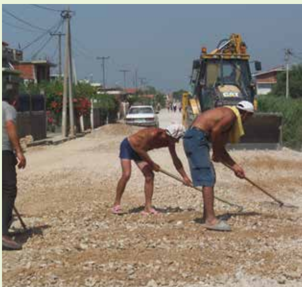
Residents working on paving and laying down the street space in informal settlements in Kamza, periphery of Tirana, Albania . © Coplan.
