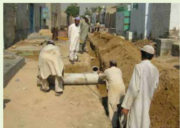
Construction of a self-help lane sewer in Gulshan-e-Zia. Street scene: during laying of sewerage pipe on self-help (background: OPP-RTI technical advisor supervises). Photo: Orangi Pilot Project.
