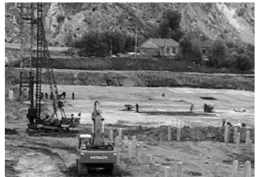
Hailin Waste Water Plant ©SHP
