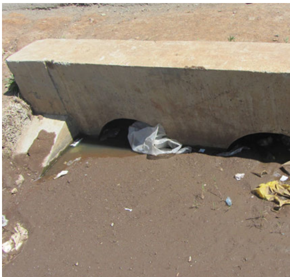
Infrastructure Management Challenges: Blocked Drainage. © Baraka Mwau
